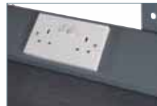
Services Duct (unwired)
